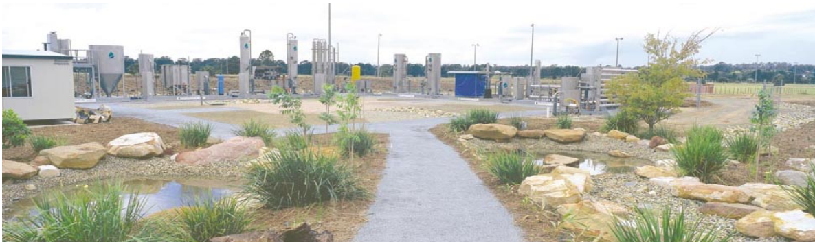
Figure 3 The Advanced Water Recycling Demonstration Plant, Brendale (Pine Rivers Shire, QLD)
