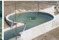
Prototype Zolotterer Gravitational Vortex Power Plant
