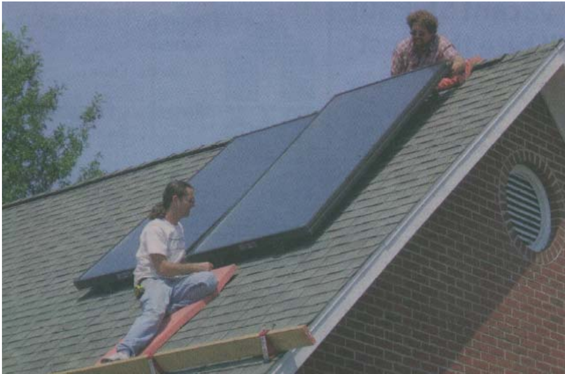
Workers from Innovative Power Systems of Minneapolis install solar panels on the garage of the newly remodeled EcoHouse on the Macalester College campus. Photo by Hi-Tech Energy Solutions
